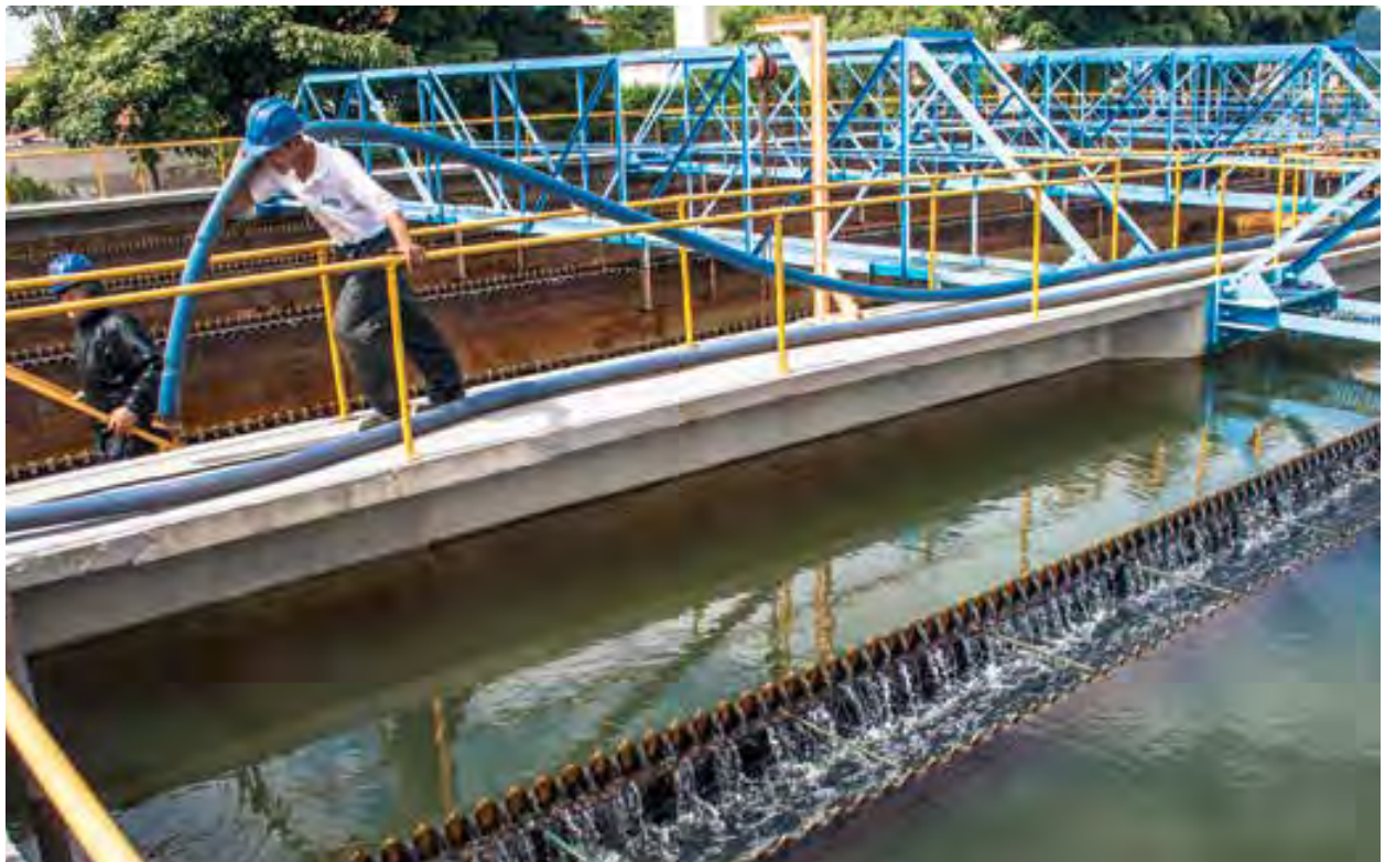
Tanks for water treatment of water and sewage in the city of Jundiaí in São Paulo, Brazil.
